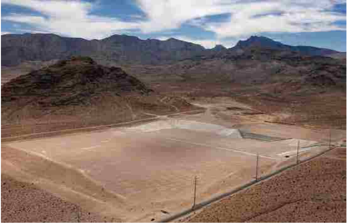
Figure 10. Ann Road Detention Basin, northeast of Las Vegas. (image courtesy of CCRFCD)
